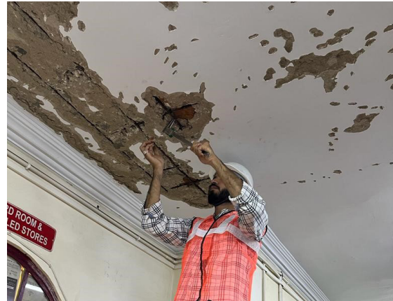
Fig.1 – Deteriorated ground floor roof slab
